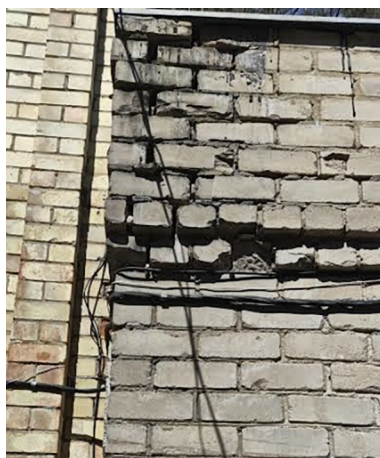
Figure 2. Defects in masonry walls due to inadequate drainage systems
