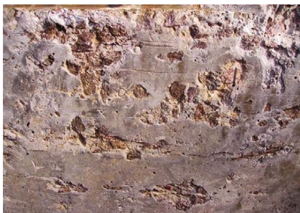
Fig. 7. External damage to the quay at the Port of Klaipeda
