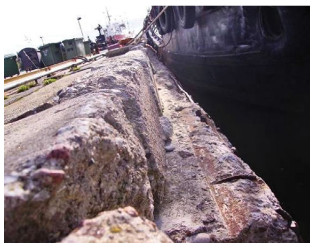
Fig. 9. Mechanical damage to the quay at the Port of Klaipeda
