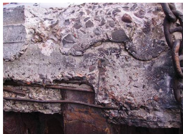
Fig. 8. Mechanical damage to the quay at the Port of Klaipeda
