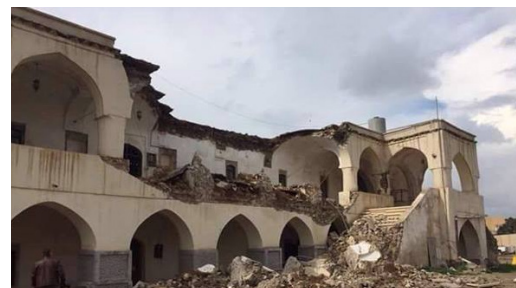
Figure 5. The collapsing part of the inside of Qishla (researcher)
