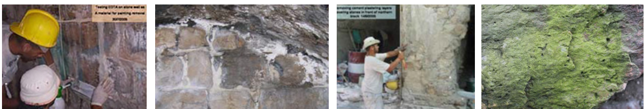
Figure 3. The problems of stone construction (Paajanen & Muinonen, 2013)
